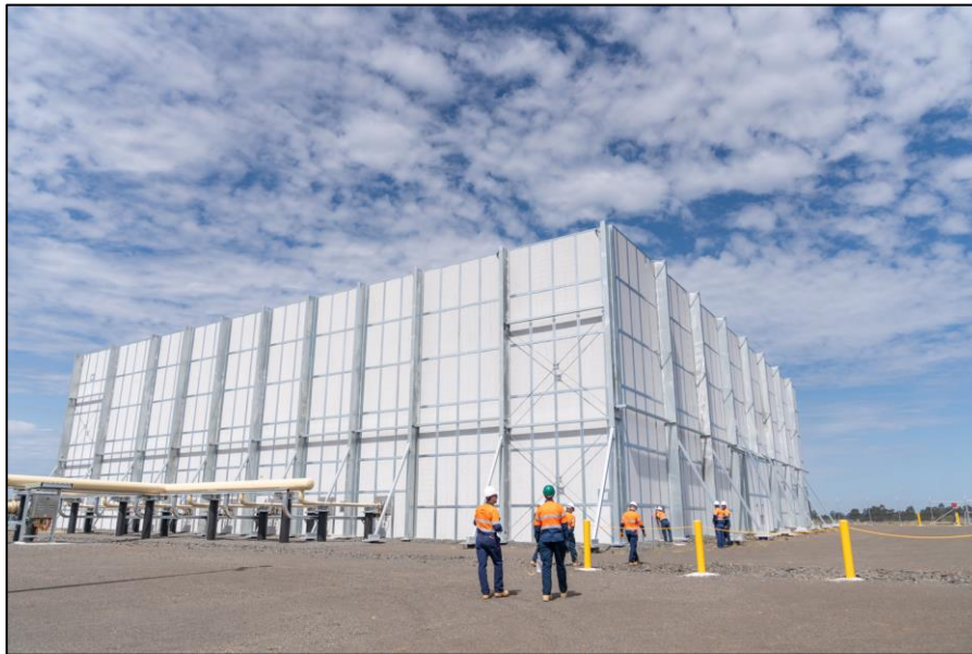
Figure 5-12 Indicative Multi-Point Ground Flare (MPGF) radiation fence
